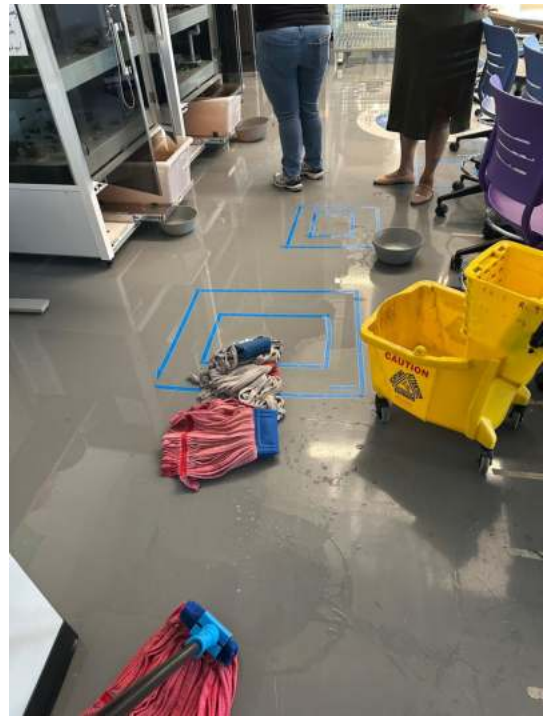
Figure C.2: The big leak
